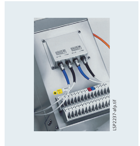
Fig. 10/6 Communication interfaces in a sloped case in a surface-mounting housing
