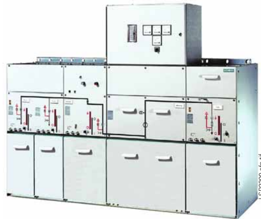
Fig. 5/13 Application in distribution switchgear
